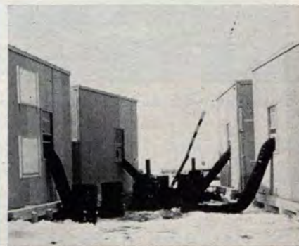
While work goes on inside, four modules get heat at the prefab plant.
