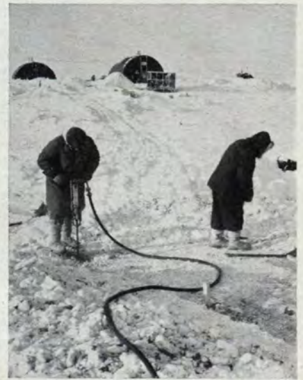
Construction workers drill holes for a foundation on a Baffin Island site.
