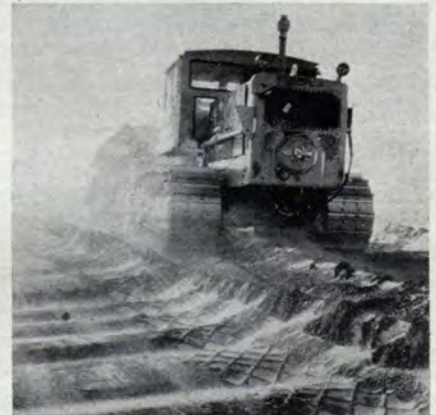
A bulldozer and scraper fight rough terrain at one of the DEW line sites.
