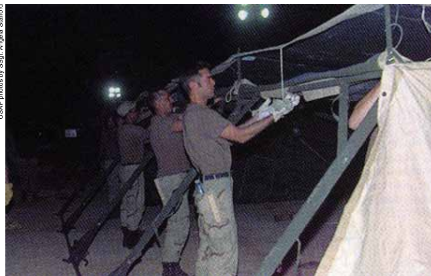
At first, USAF RED HORSE units did most of the heavy lifting. They handled the equivalent of 25 C-5 loads of lumber, canvas, generators, and other supplies so that arriving troops would have places to eat, sleep, and do their work.
