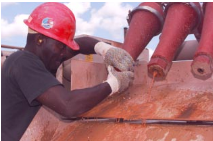
TSgt. Willie Daniels, 307th RED HORSE Squadron—a construction and engineering unit from Barksdale, La.—works on equipment that cleans sand out of a well. USAF personnel from Barksdale and Kelly AFB, Texas, went to Belize from January through March for New Horizons 2000, an annual humanitarian mission.
