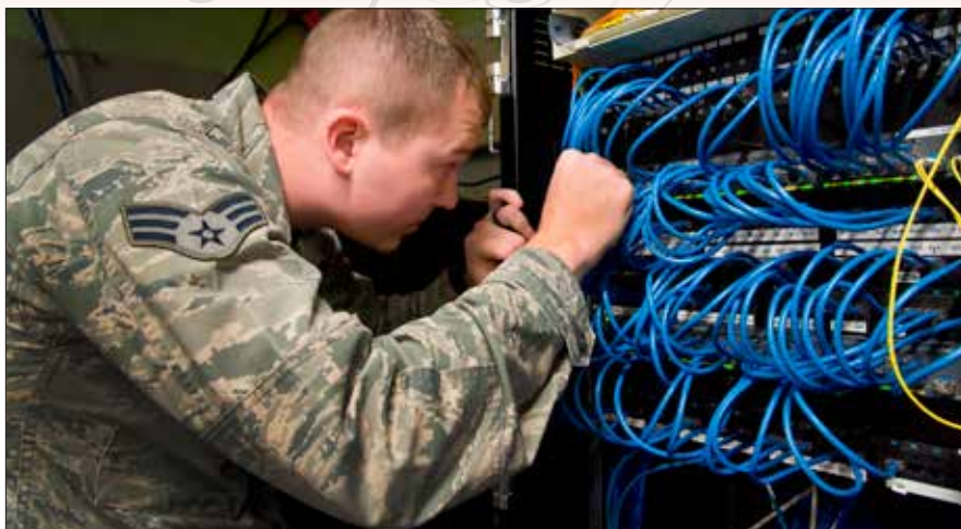
SrA. Gene Kellenberger, a cyber systems operations journeyman, reconnects cables at Dover Air Force Base in Delaware. Gen. David Goldfein, USAF Chief of Staff, says the volume of data collected outpaces the capacity for analysis.
